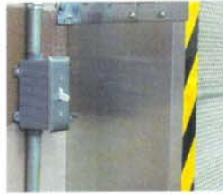
Metal sheeting covers the side of the guide tracks to provide a secure seal.
